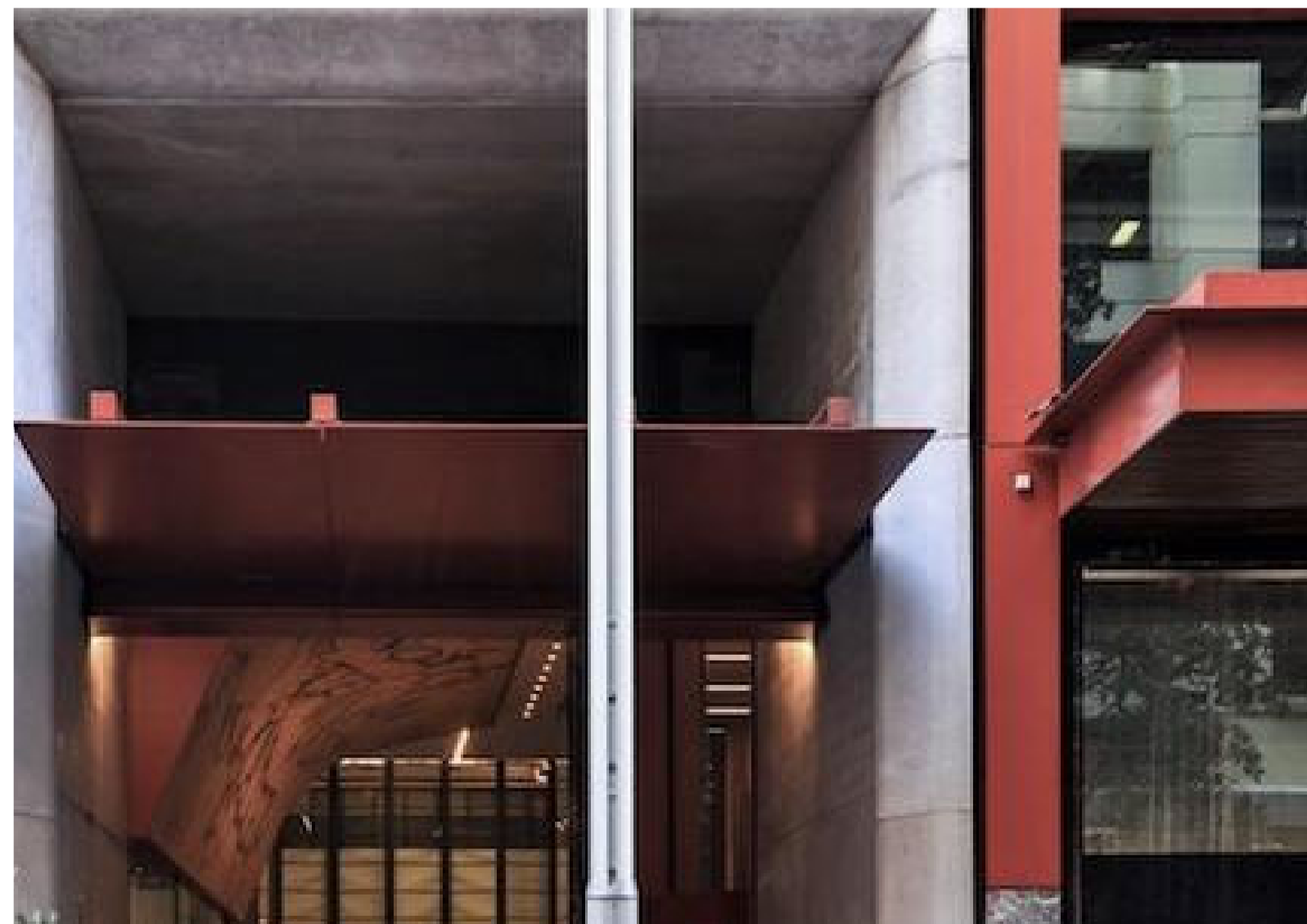
METAL FINISH (MF1) POWDER COAT STEEL AND ALUMINIUM (INTERPON D2525 SABLE CORTEN)
